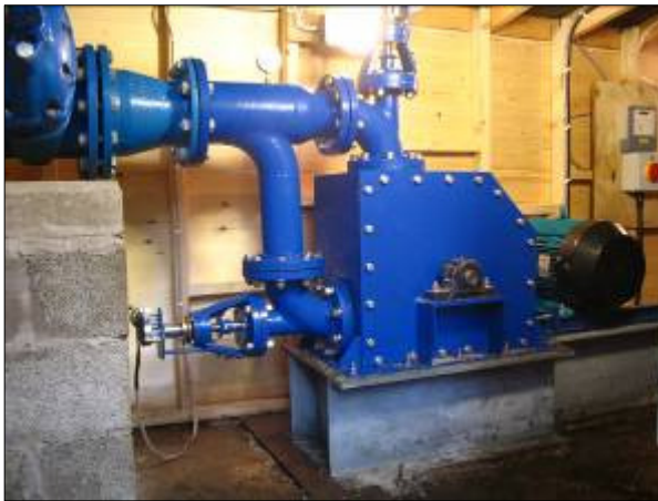
Micro-hydro - Derwentwater Youth Hostel, Barrow House, Borrowdale, Keswick
